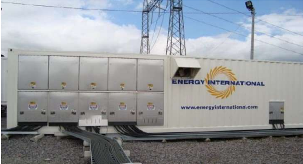
Figura 25 Tablero de control 13.8 Kv
