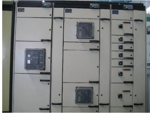
Motor Control Center / Power Center
