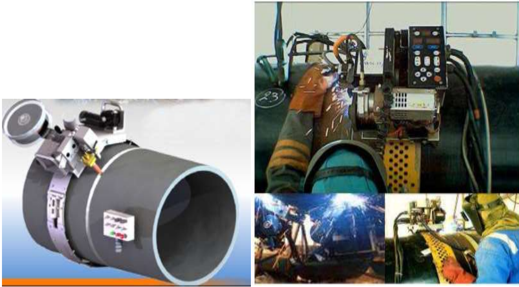
FIGURA 9. WELDING HEAD UNITS (WHU)
